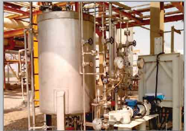
Chemical Injection Package
